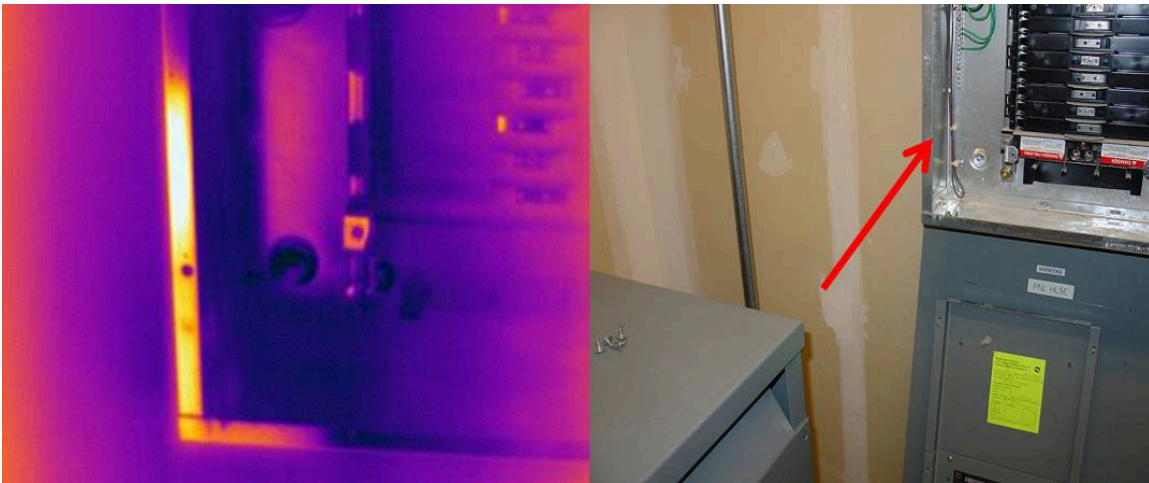
Figure 1 - Reflection of transformer in panel
